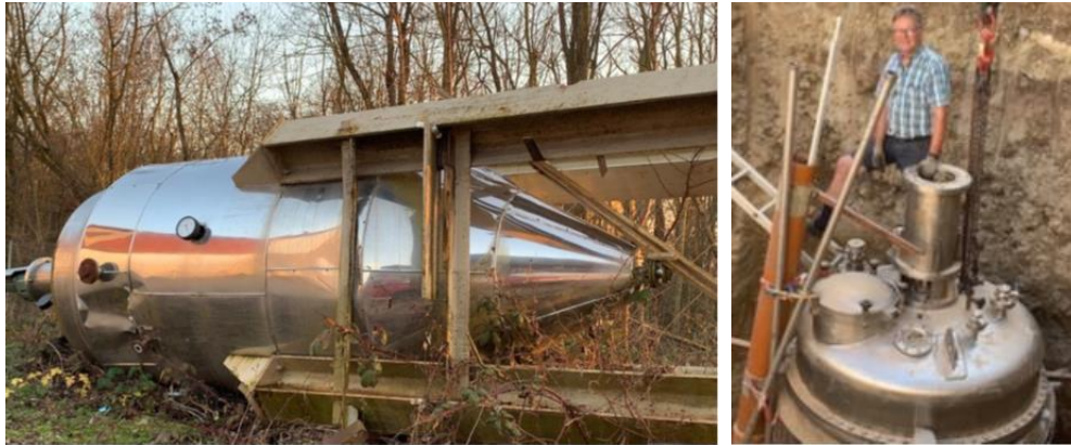
Figure 34 Stainless steel container with temperature insulation before and after installation under-ground (photos: D. Gräf)
